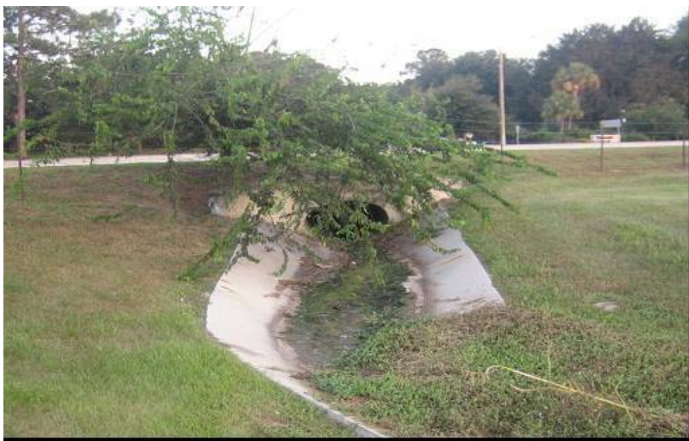
Figure 2. A concrete ditch with soil and plant hindering storm water flow (requires cleaning)
